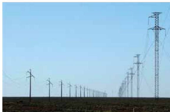
Our transmission network is a key consideration for integrating renewable energy generation in Australia. Source: Arthur Mostead
